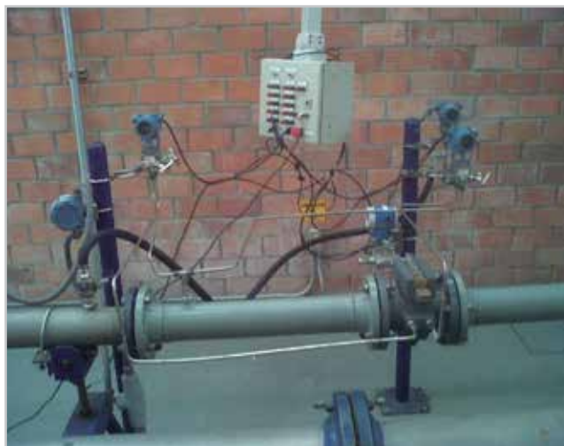
Figure 3. CIATEQ 4" water flow facility with an orifice meter diagnostic ready.
