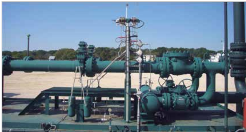
Figure 29. Dual chamber 10" orifice meter run with the system installed.
