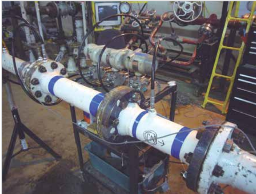
Figure 20. Air blow down facility with a 4", 0.5β paddle plate orifice meter installed with a 6D downstream pressure port for diagnostics.
