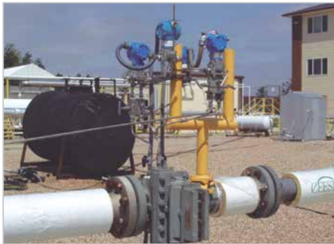
Figure 26. 4" Orifice meter with downstream pressure port at the CEESI wet gas flow facility.
